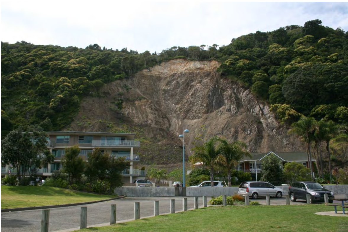
Figure 8.8: Large structurally-controlled landslide behind No. 33 Muriwai Drive. The complexly deformed greywacke of the Whakatane Mélange is overlain by the light coloured Upper Ohope Beds.
