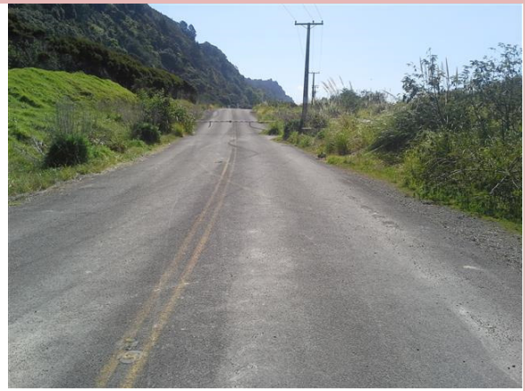
Looking west along McPherson St towards higher ground and gate that requires relocation.
