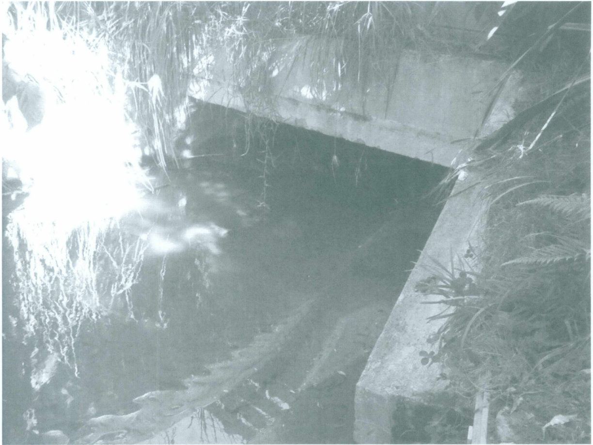
Image 4: The Waimea Stream culvert under Pakeha Street showing some silt build up - evidence the culvert has been set a little low.
