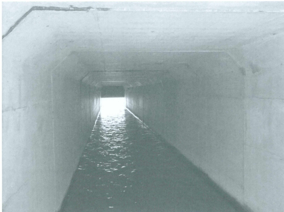
Image 3 : The culvert under the debris bund discharging to the Waitepuru watercourse that flows through the town - looking upstream to the temporary choke plate.
