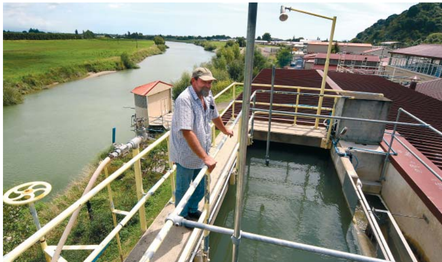
The water treatment plant.
