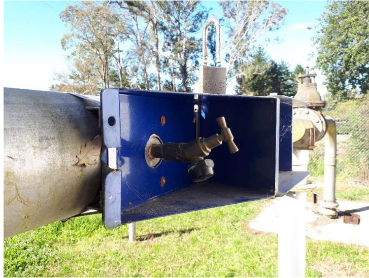
Figure 8: View of opened sample box on pipework from bore
