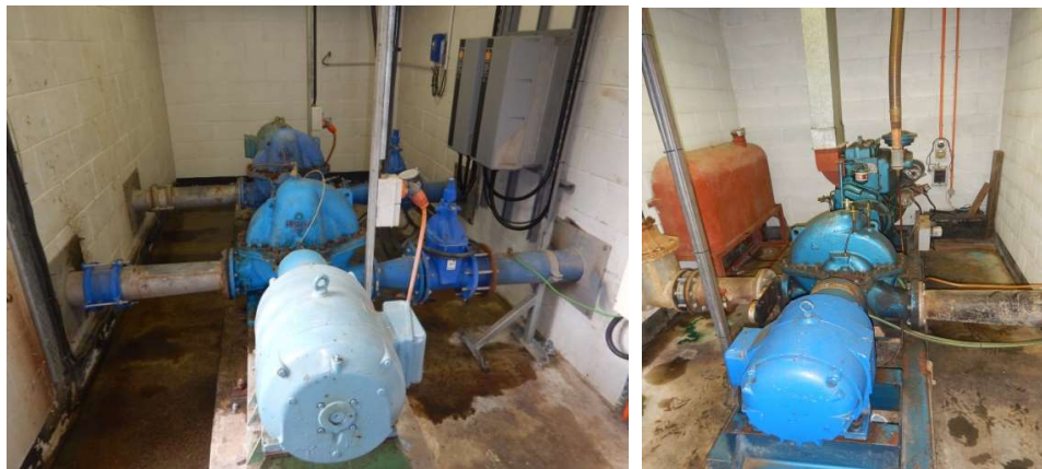
Figure 6: Suction Tank (Top), Two High-Lift pumps (Bottom Left) and Diesel pump with diesel storage (Bottom Right)
