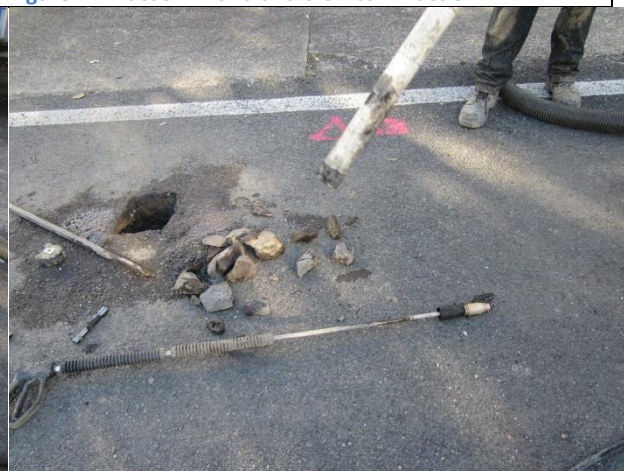
Figure 24. Vacuum debris and fill recovered
