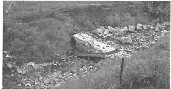
Works in stream beds such as building bridges or dams may need a consent
