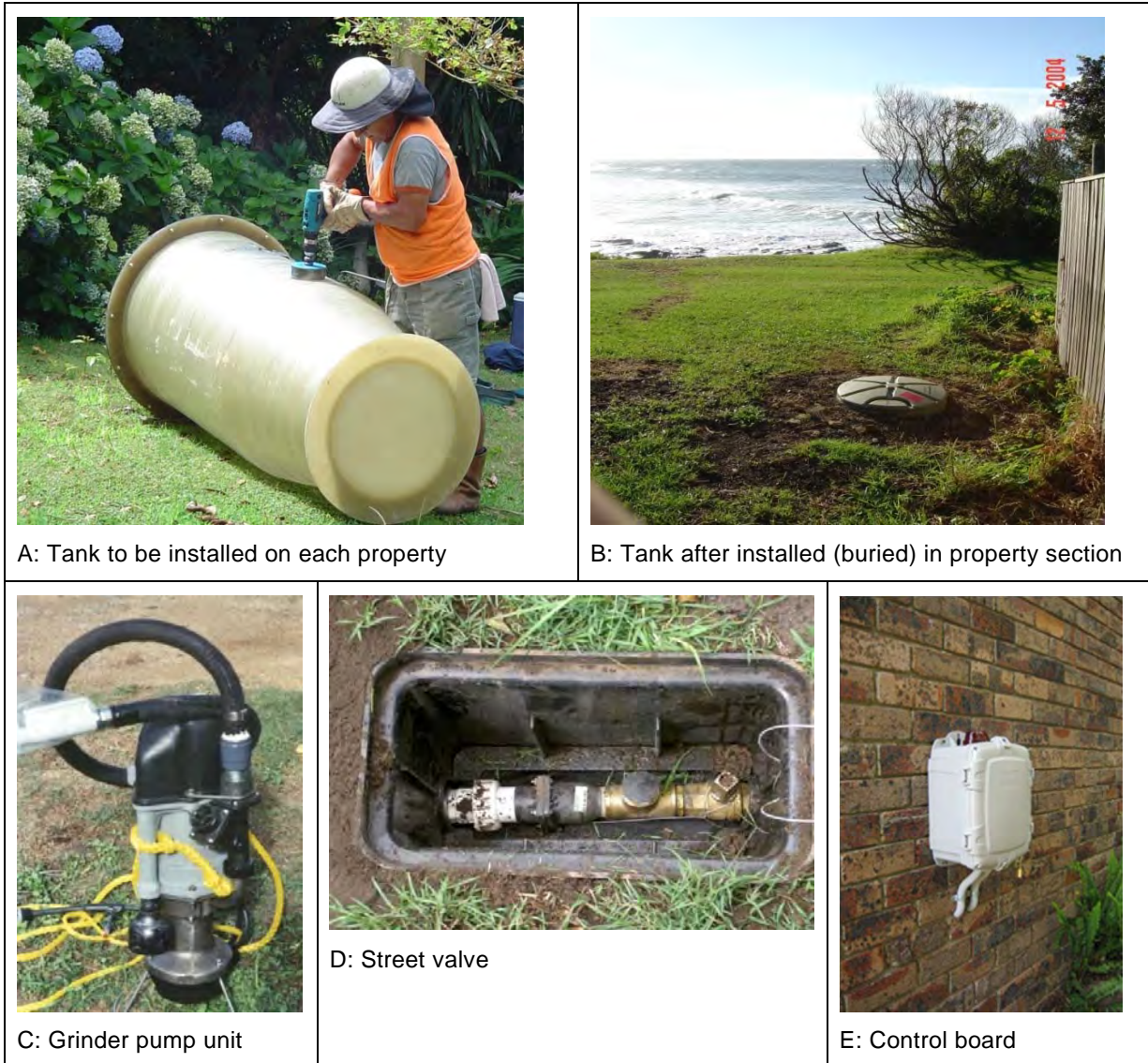
Figure 5-3: Photographs (A – E) showing a typical Low Pressure Grinder Pump System
