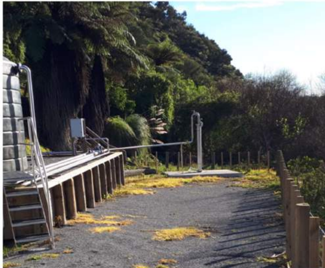
Figure 4: Tahuna Road Water Treatment Plant borehead
