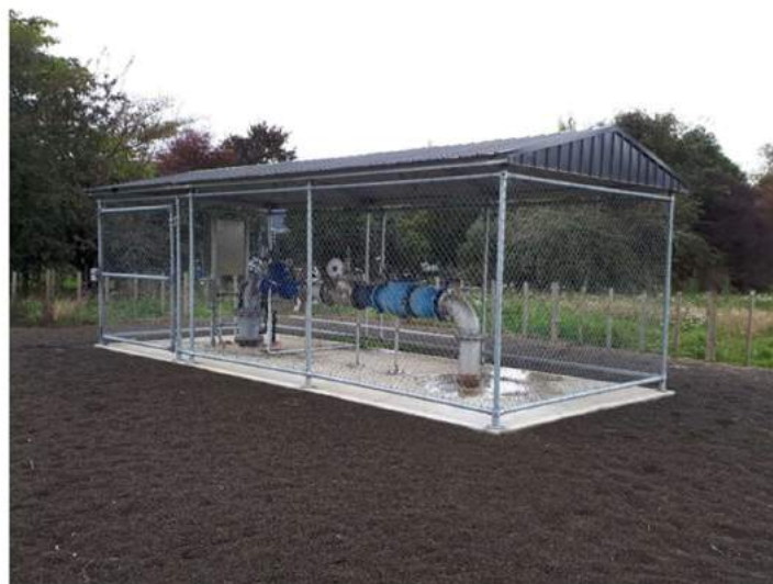
Figure 3: Paul Road Borehead and security enclosure
