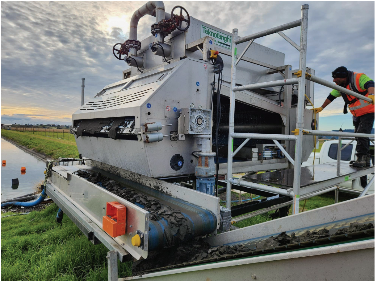
The belt press in operation at the Whakatāne wastewater treatment plant
