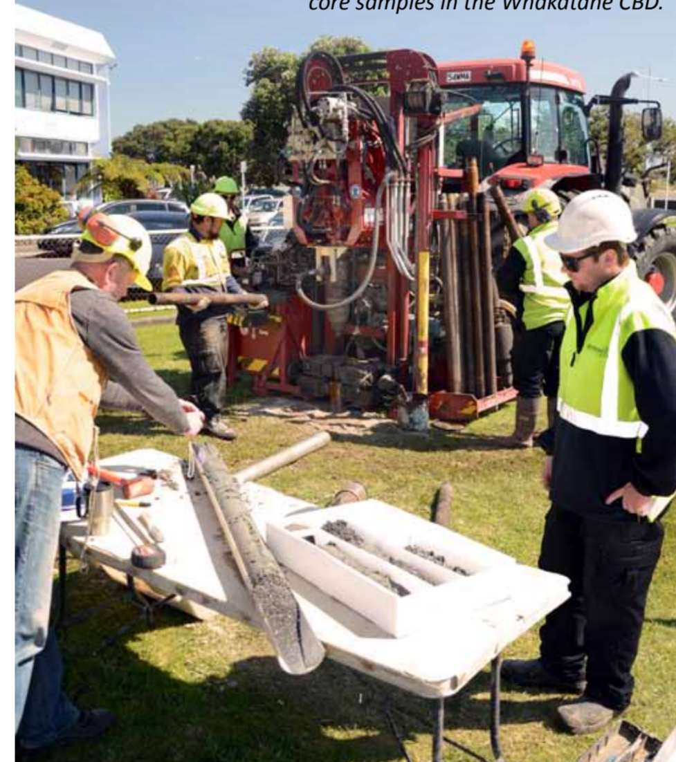
Ian Brown Associates Ltd staff taking core samples in the Whakatāne CBD.
