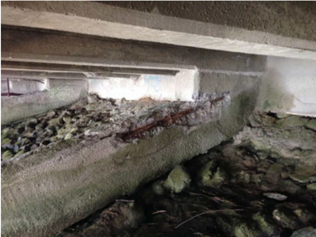
Photo A34 - spalling of raker beam at A6
