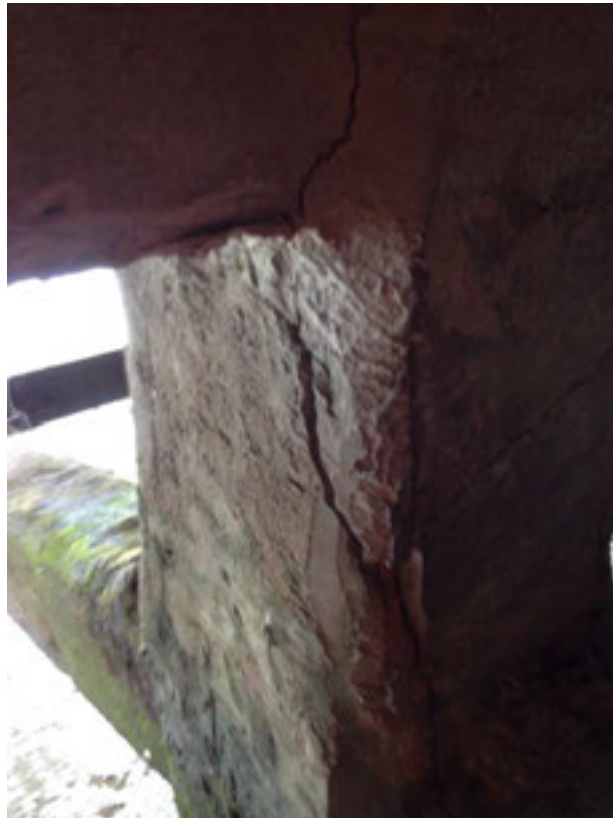
Photo A27 - Cracking of pile at A4
