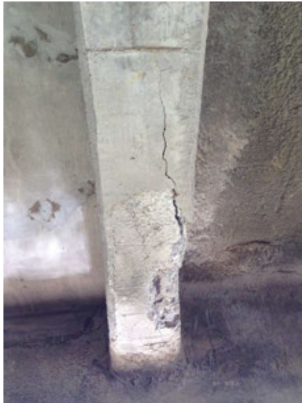
Photo A07 - beam cracking / spalling between A1 and A2
