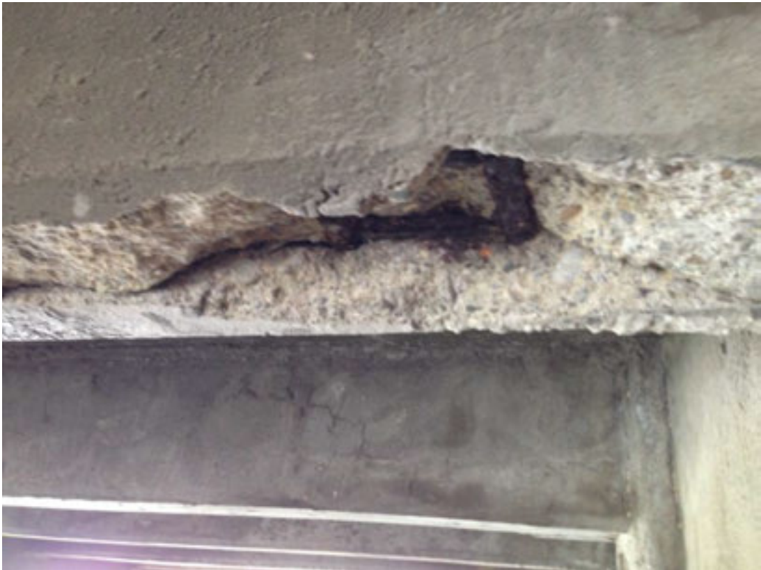
Photo C09 - spalling of beam
