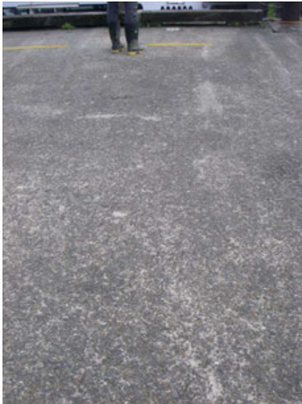
Photo T06 - cracking in slab (1940 section)
