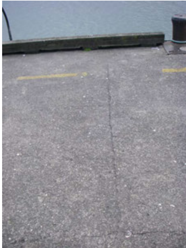
Photo T09 - cracking in slab (1919 section)
