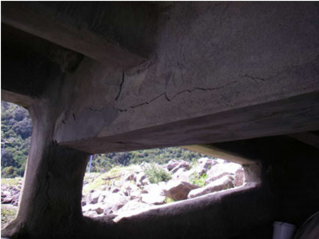
Photo A03 - beam cracking between A1 and A2
