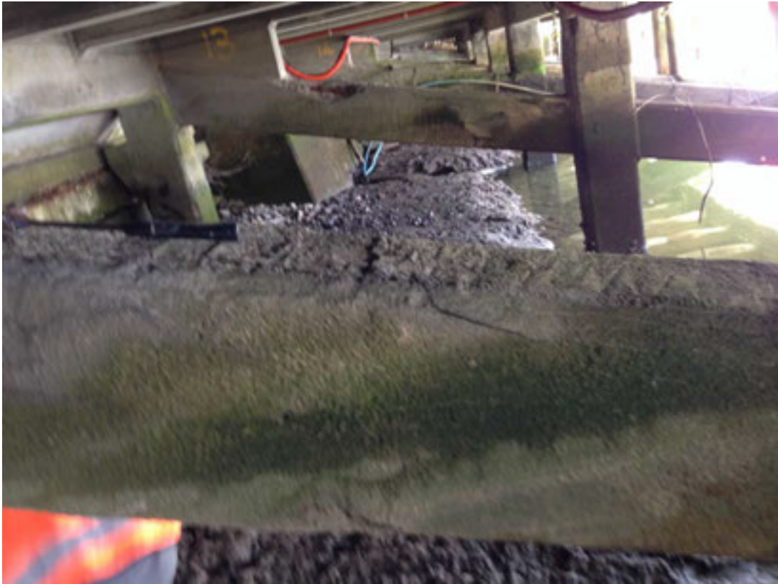
Photo B12 - spalling of raker beam at B12
