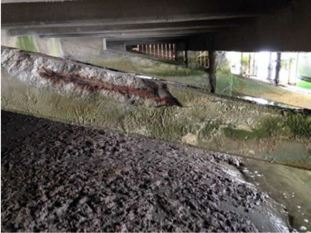
Photo C08 - cracking of raker at C6
