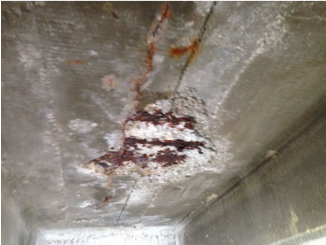
Photo C06 - spalling of slab
