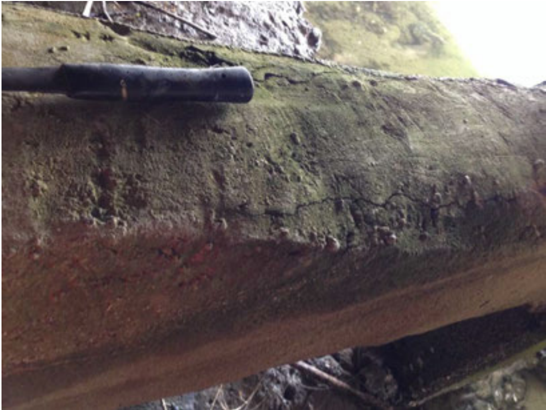
Photo B10 - cracking of raker beam at B9
