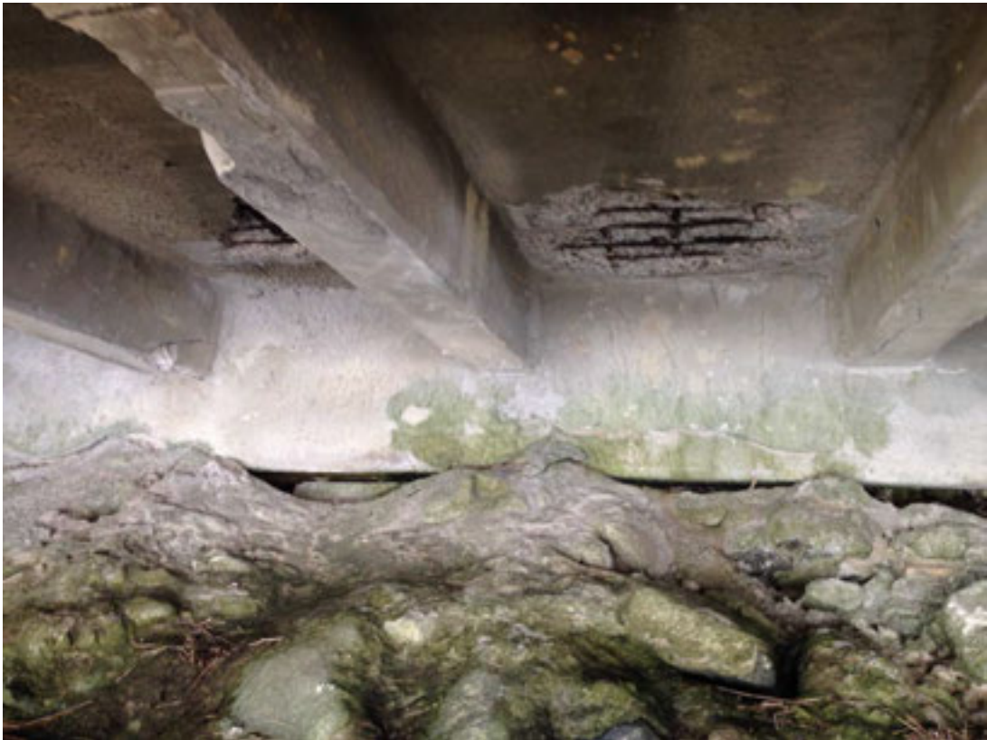
Photo A13 - spalling of slab between A2 and A3
