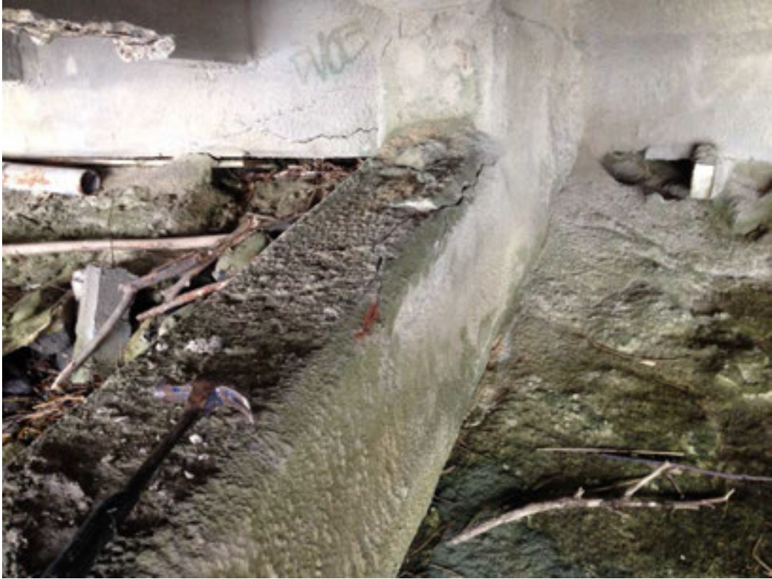
Photo A26 - cracking of raker beam at A4
