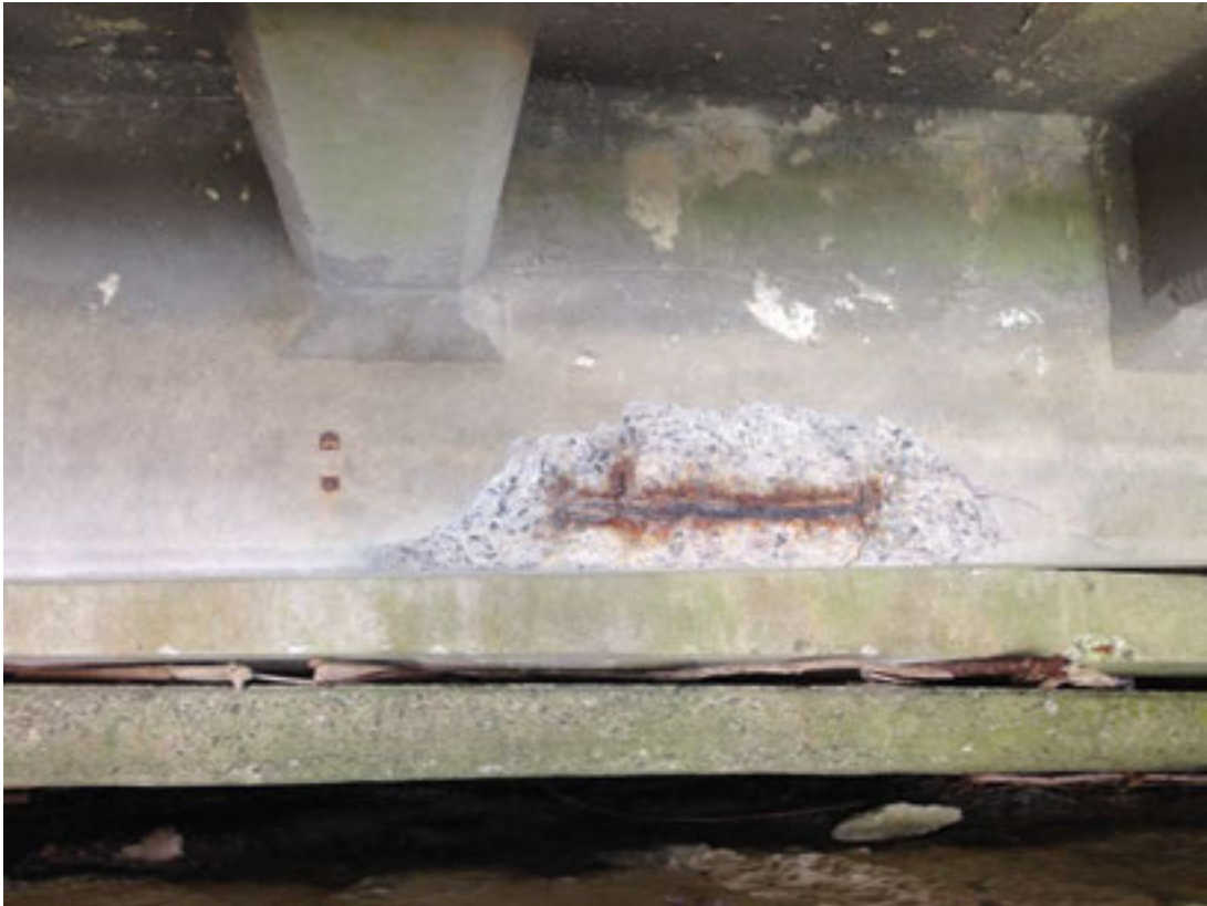
Photo B16 - spalling of rear beam between B15 and B16
