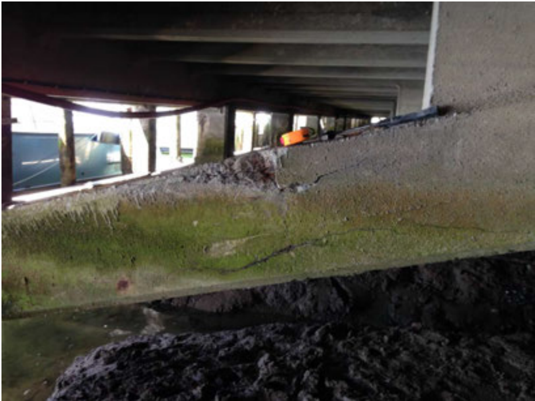
Photo B15 - spalling of raker beam at B13
