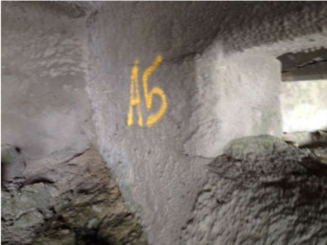
Photo A28 - Cracking at A5
