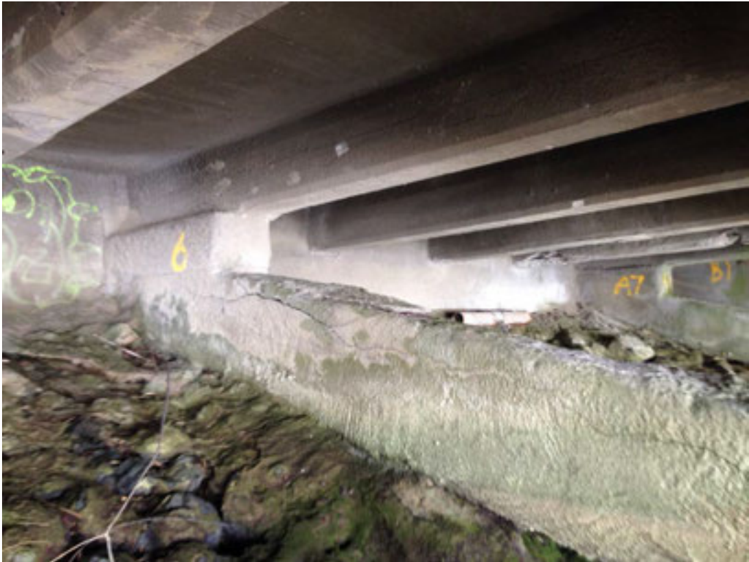
Photo A32 - cracking of raker beam at A6
