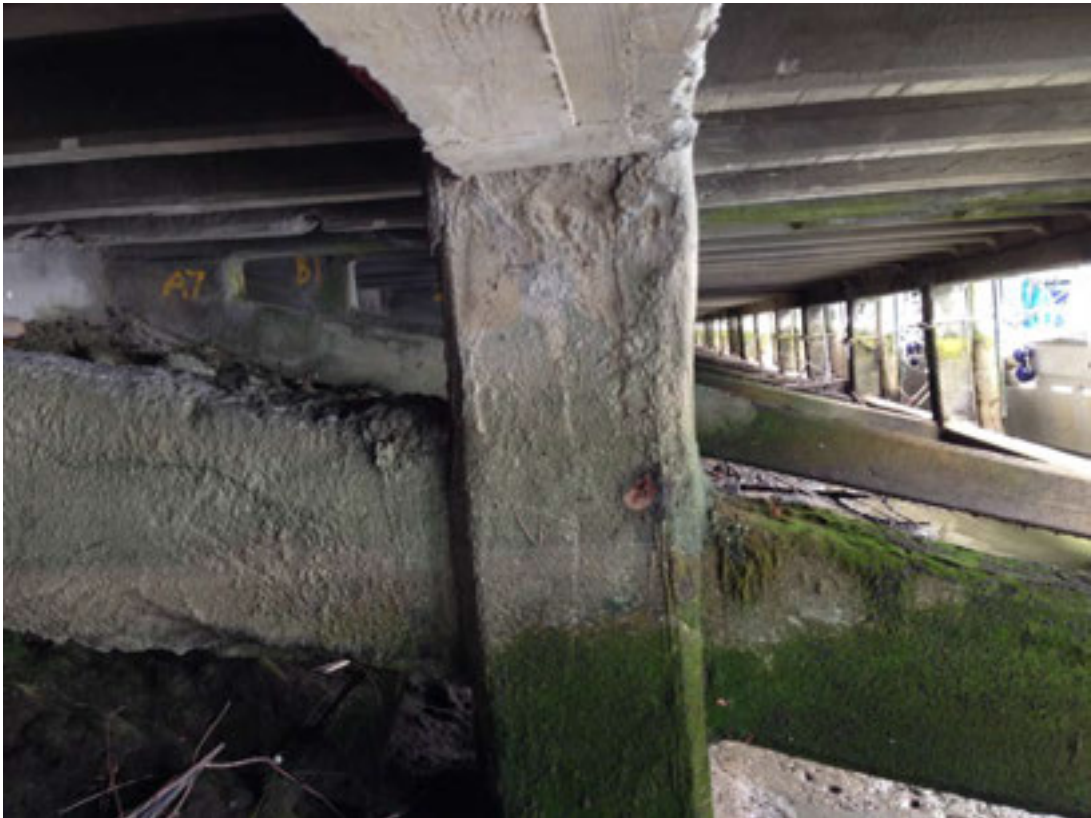
Photo A33 - cracking of raker beam at A6
