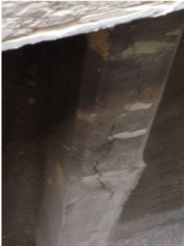
Photo A19 - Cracking of beam between A3 and A4
