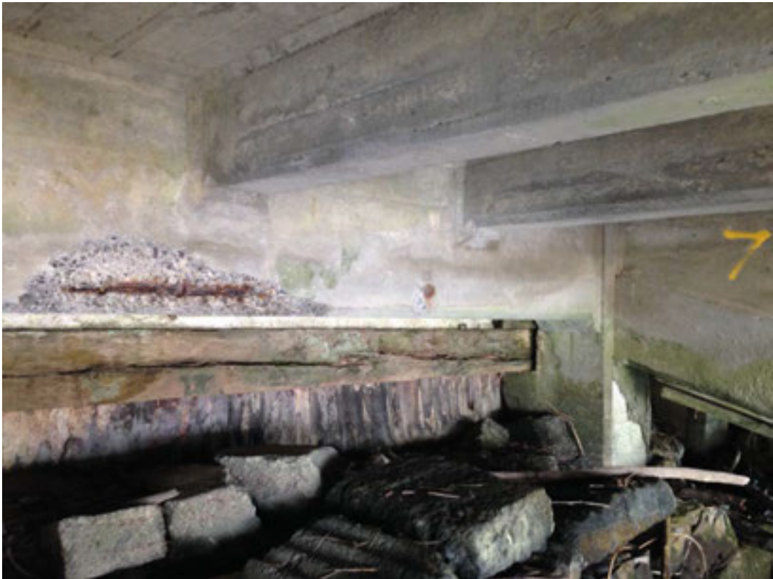
Photo B09 - spalling of rear beam between B6 and B7
