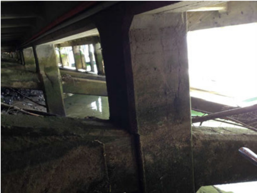
Photo B07 - Pile cracking at B5
