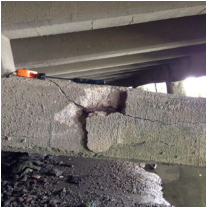
Photo C01 - cracking in beam at C2
