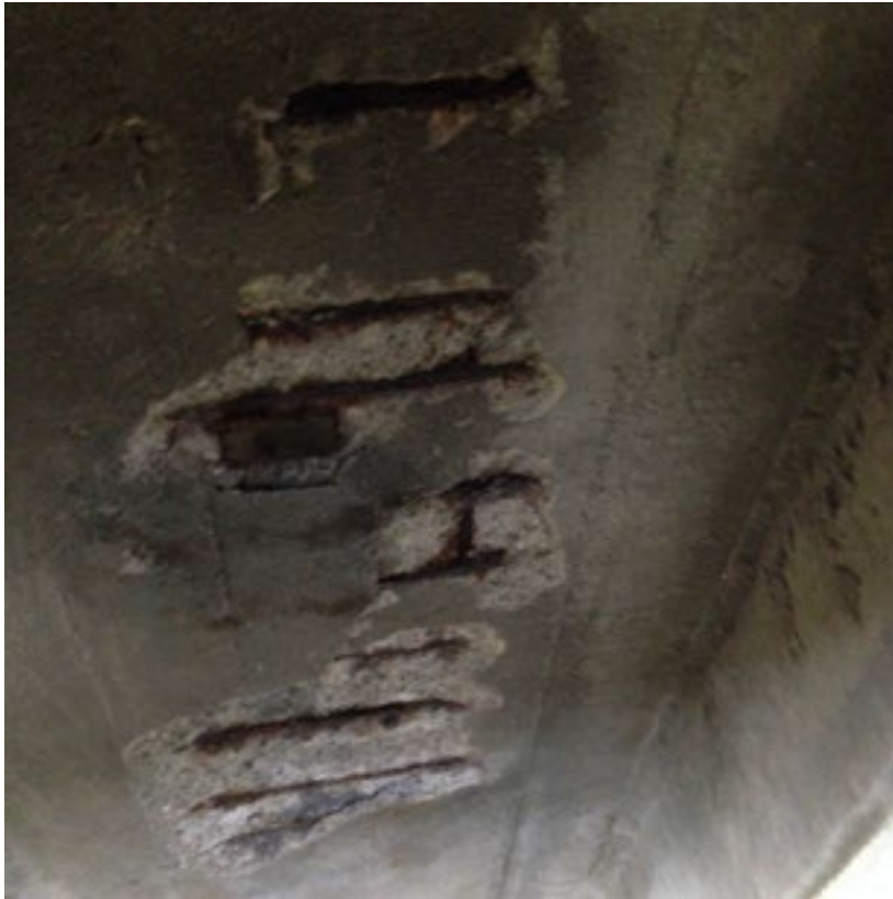
Photo C02 - slab spalling between C2 and C3
