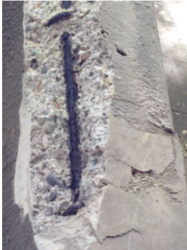
Photo A20 - spalling of beam between A3 and A4
