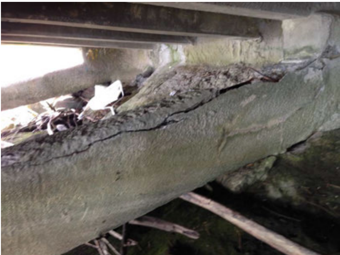
Photo A11 - spalling of raker beam at A2
