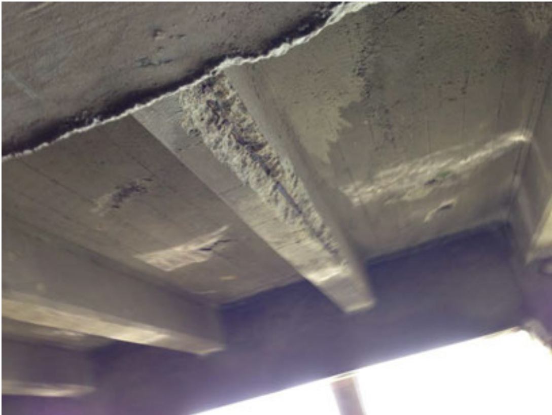
Photo C03 - beam spalling between C1 and C2
