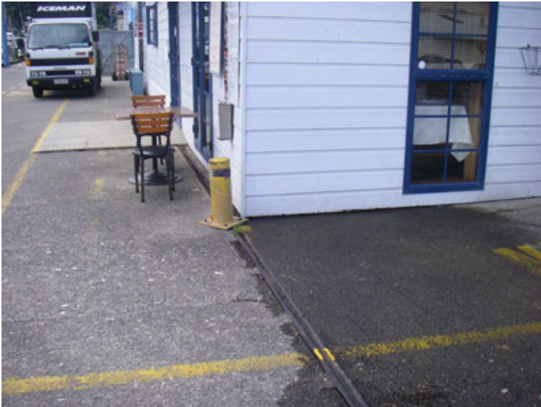
Photo T12 - cracking in slab (1919 section)
