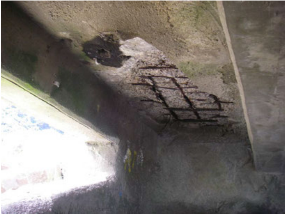
Photo A04 - slab spalling between A1 and A2
