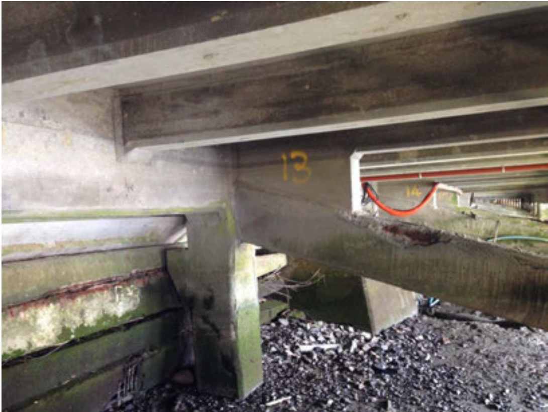
Photo B14 - spalling of raker beam at B13
