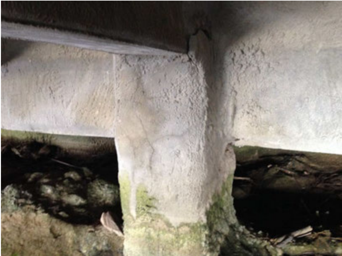
Photo C04 - cracking of pile repair
