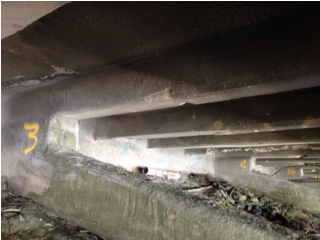
Photo A17 - spalling of beam at A3
