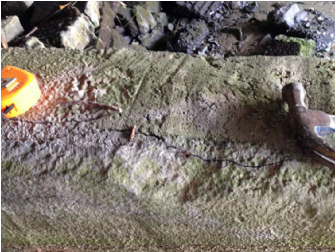
Photo B08 - Cracking of raker beam at B6
