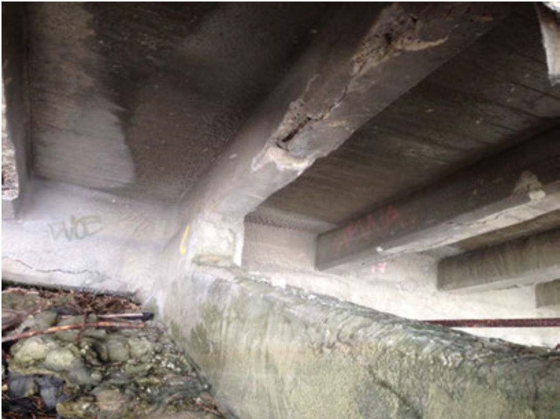
Photo A23 - spalling of beam at A4
