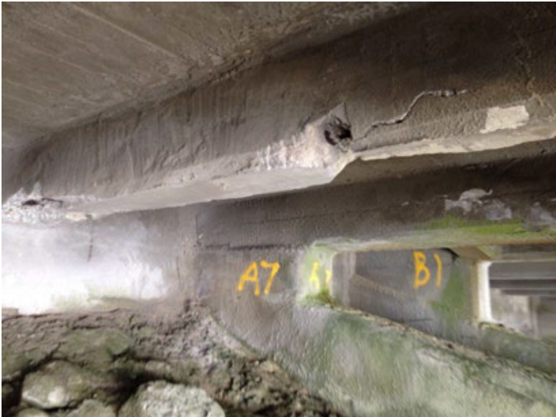
Photo A35 - Spalling of beam between A6 and A7
