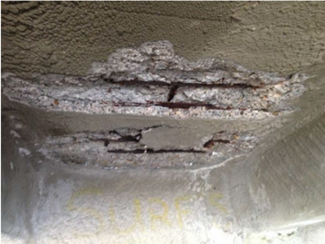
Photo A06 - slab spalling between A1 and A2
