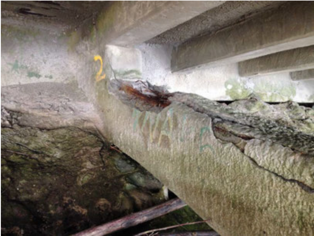
Photo A10 - spalling of raker beam at A2
