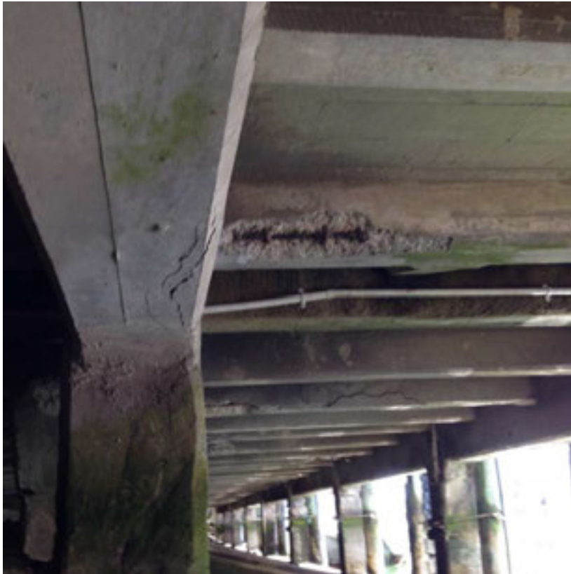
Photo B18 - cracks in beams at B15
