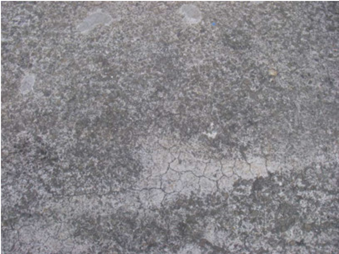
Photo T04 - cracking in slab (1936 section)
