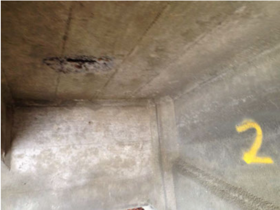
Photo B04 - slab spalling between B1 and B2
