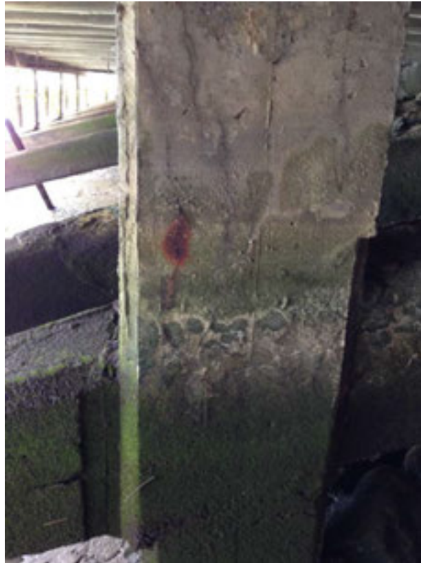
Photo B02 - Staining at B1
