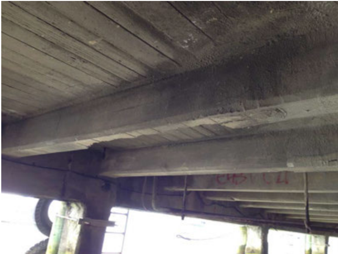
Photo A31 - spalling of beam between A5 and A6
