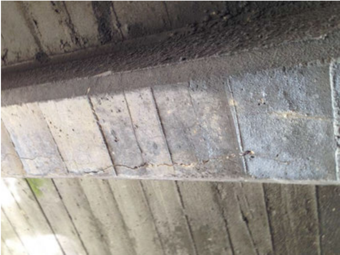
Photo A36 - cracking of beam between A6 and A7
