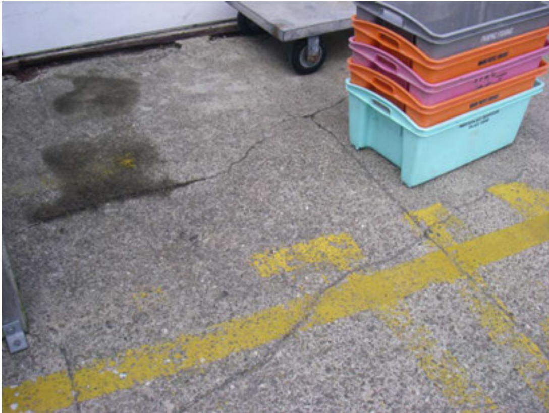
Photo T11 - cracking in slab (1919 section)
