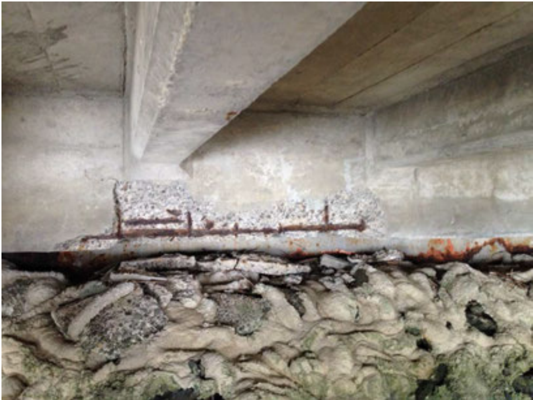
Photo B05 - rear beam spalling between B2 and B3
