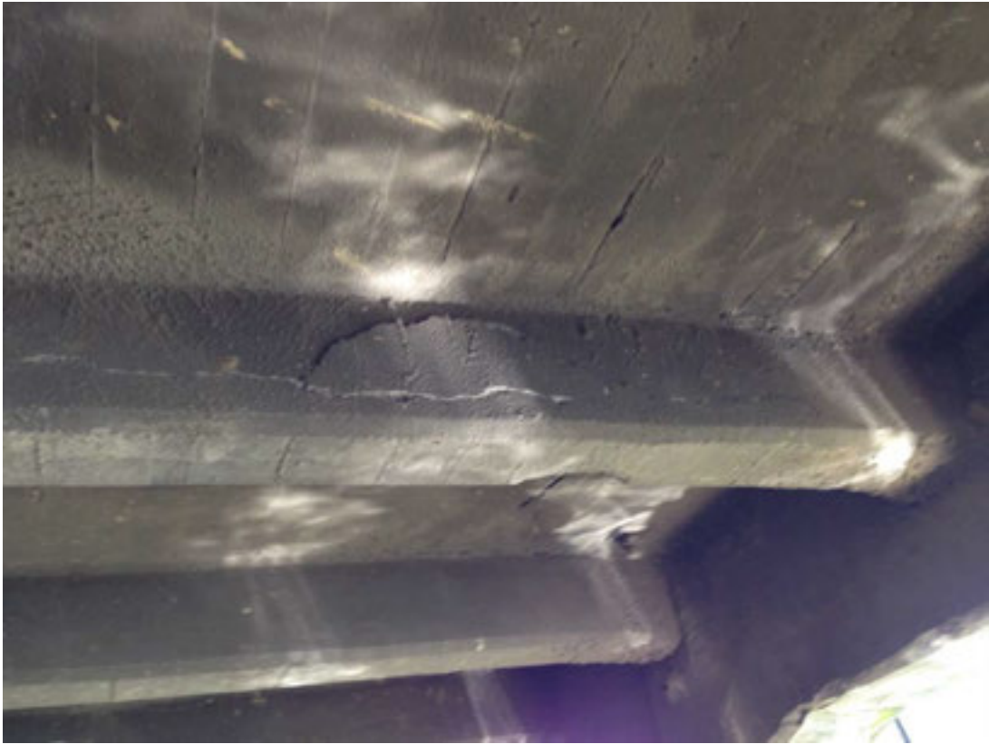
Photo A16 - cracking of beam between A2 and A3
