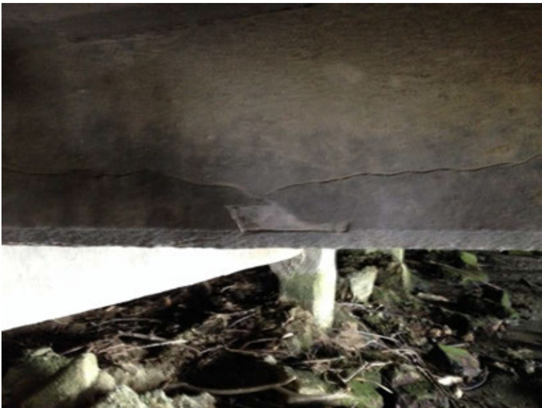
Photo C05 - cracking of beam
