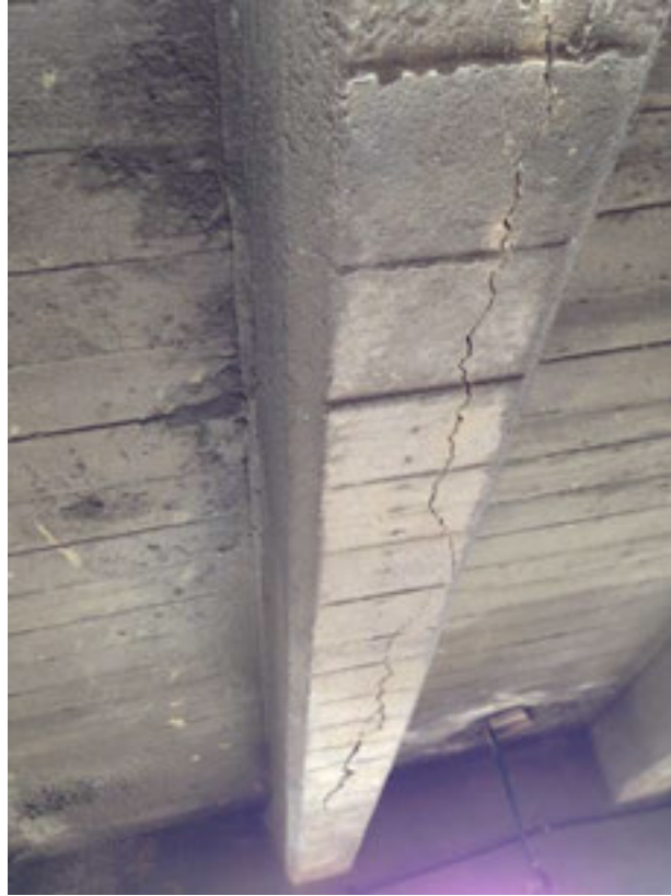
Photo A30 - cracking of beam between A5 and A6
