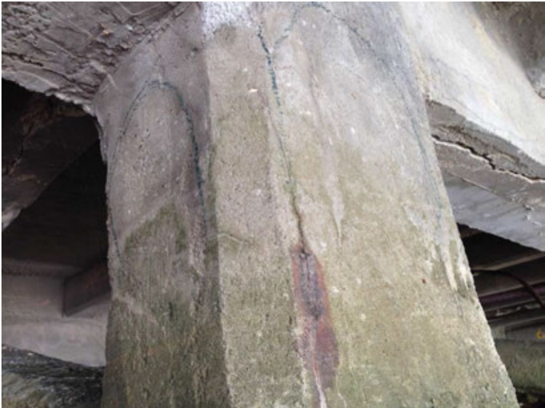
Photo A25 - Pile cracking at A4
