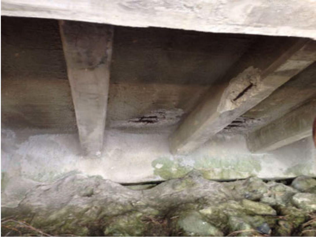
Photo A14 - spalling of slab between A2 and A3
