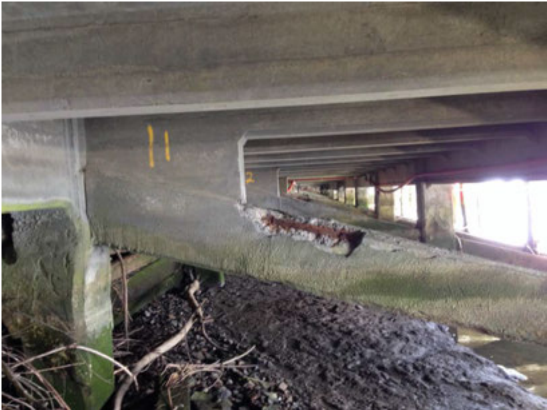
Photo B11 - spalling of raker beam at B11
