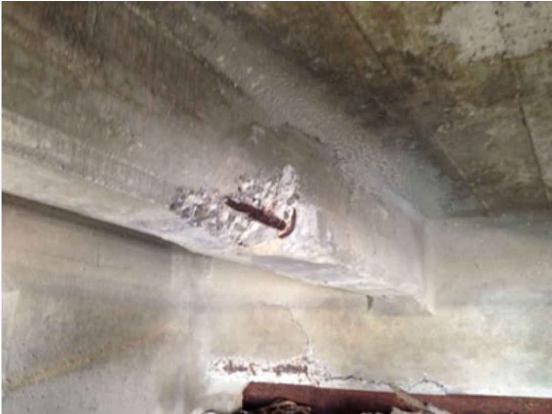
Photo B06 - beam spalling between B4 and B5
