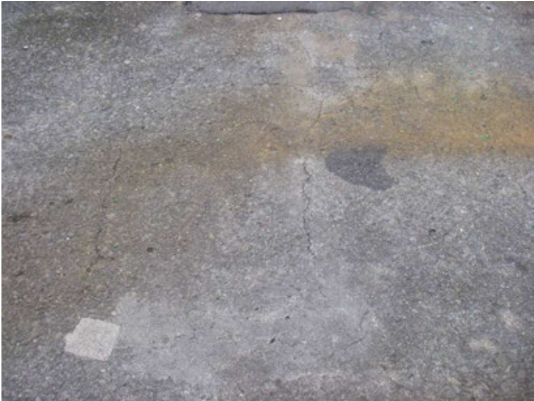
Photo T03 - cracking in slab (1936 section)
