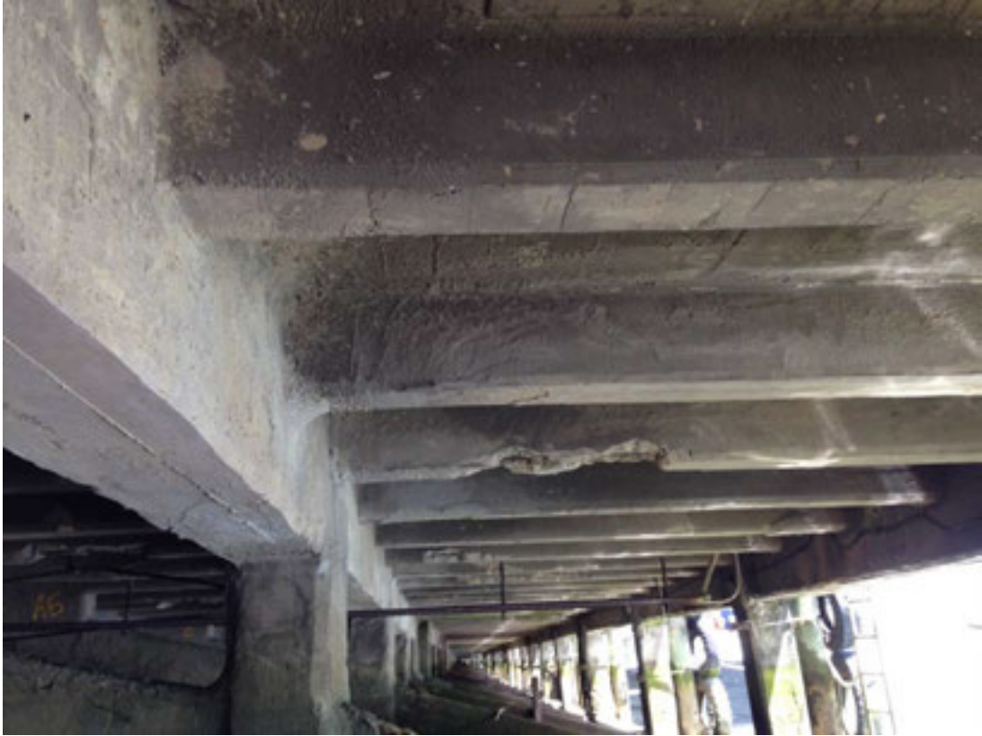
Photo A22 - spalling of beam at A4
