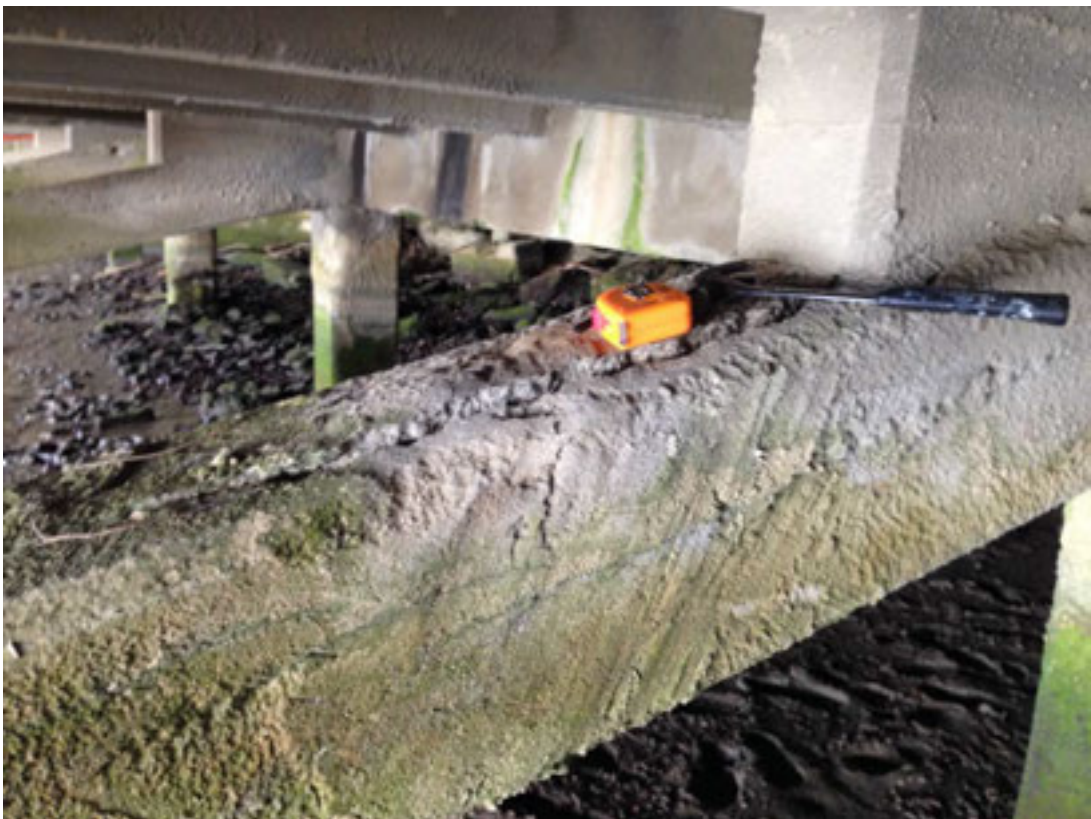
Photo C07 - cracking of raker at C7
