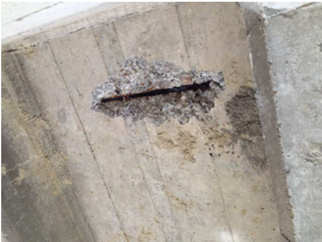
Photo B03 - slab spalling between B1 and B2
