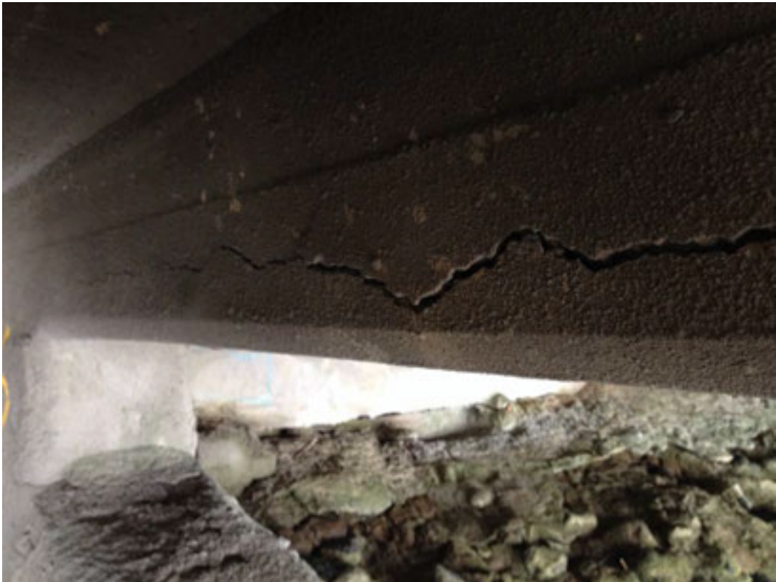
Photo A29 - Cracking of beam at A5
