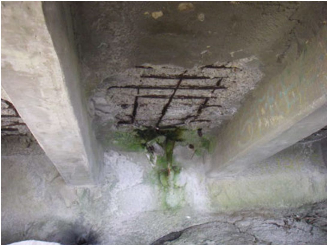
Photo A05 - slab spalling between A1 and A2
