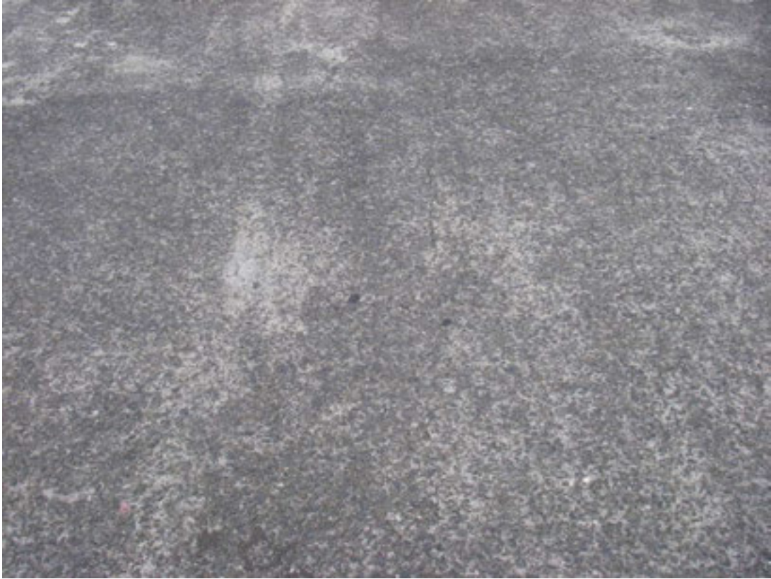
Photo T05 - cracking in slab (1940 section)
