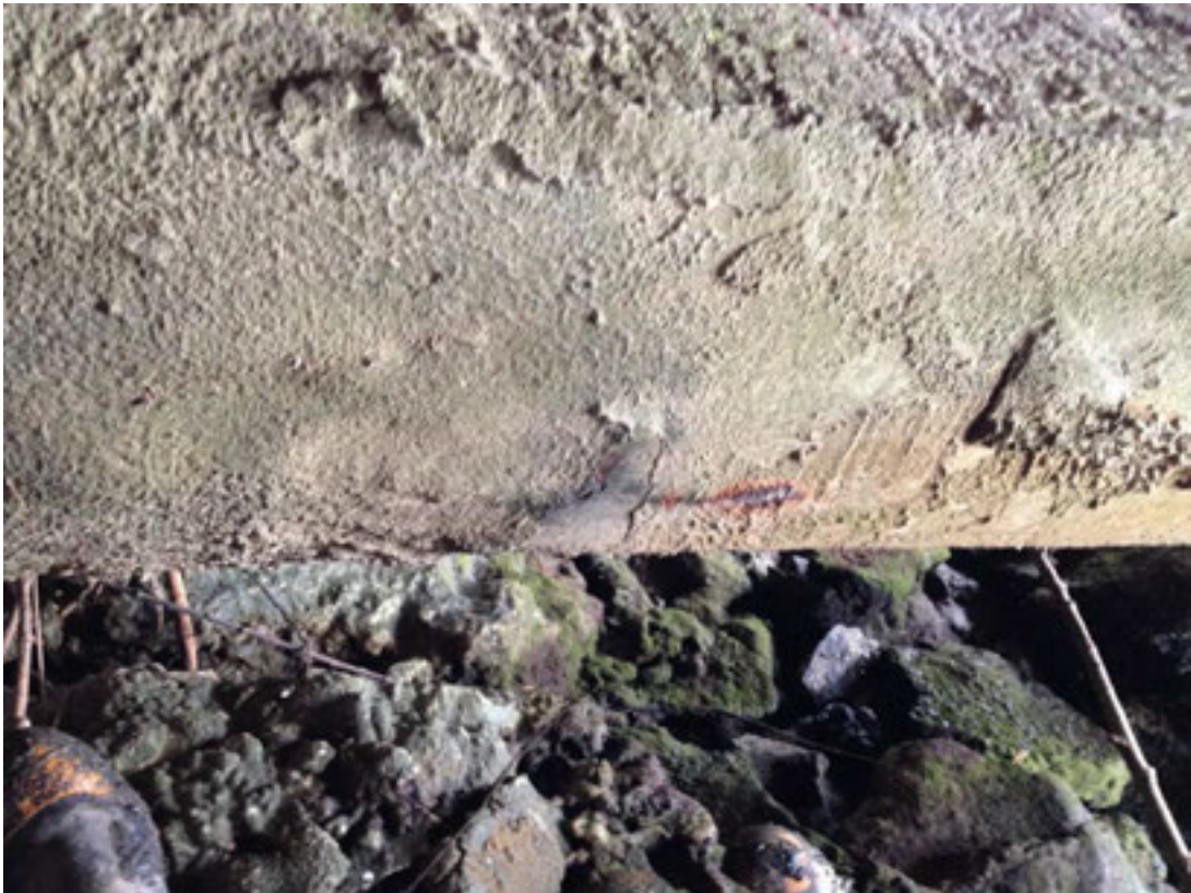
Photo B01- Staining at B1
