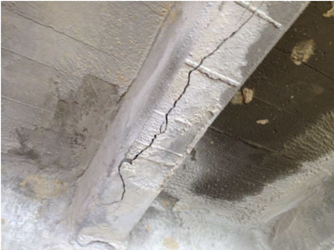
Photo A15 - cracking of beam between A2 and A3
