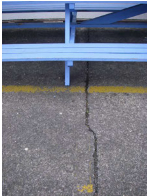
Photo T10 - cracking in slab (1919 section)
