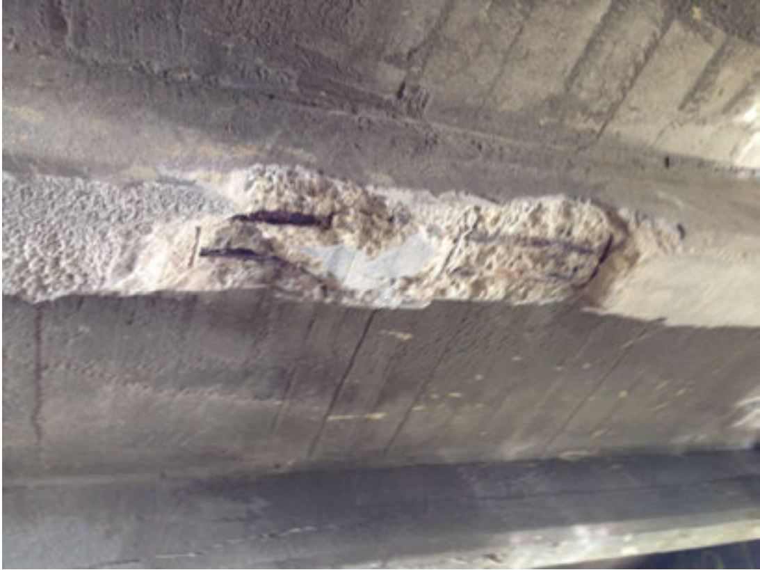
Photo A24 - spalling of beam at A4
