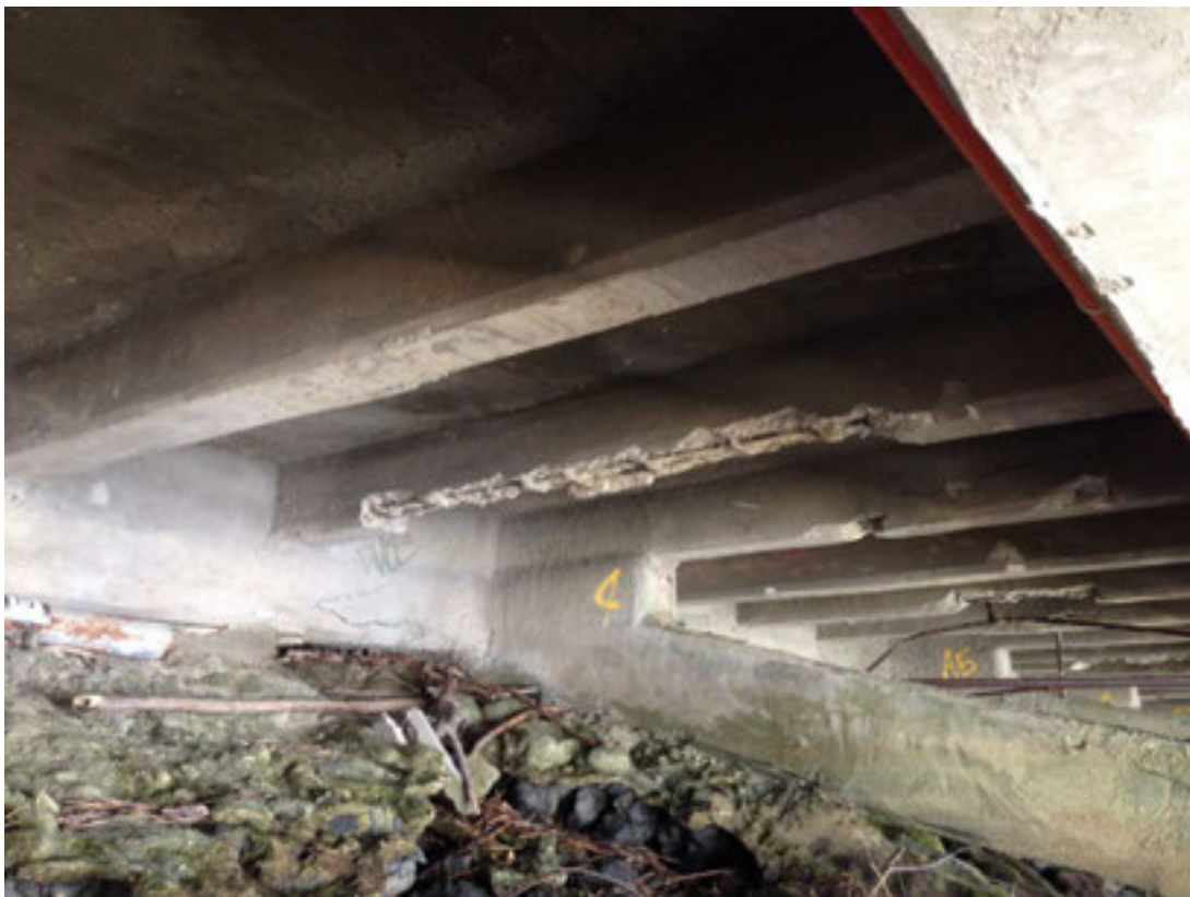
Photo A21 - spalling of beam between A3 and A4
