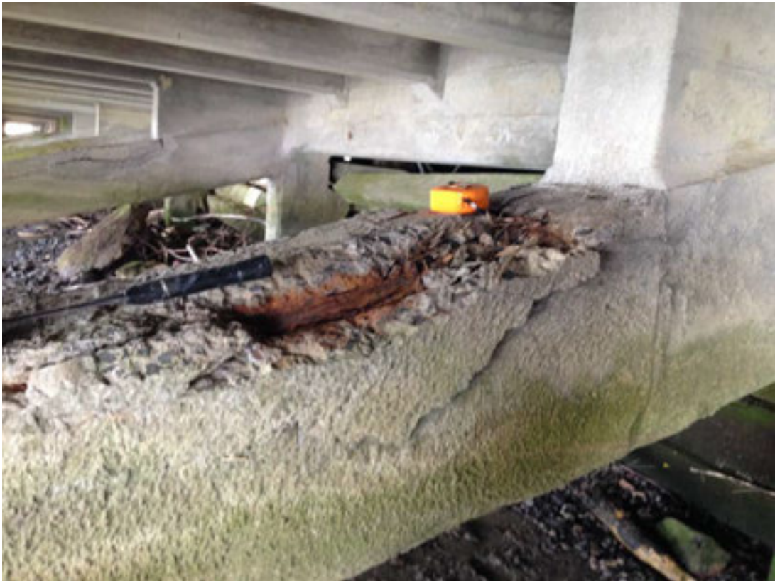
Photo B13 - spalling of raker beam at B12
