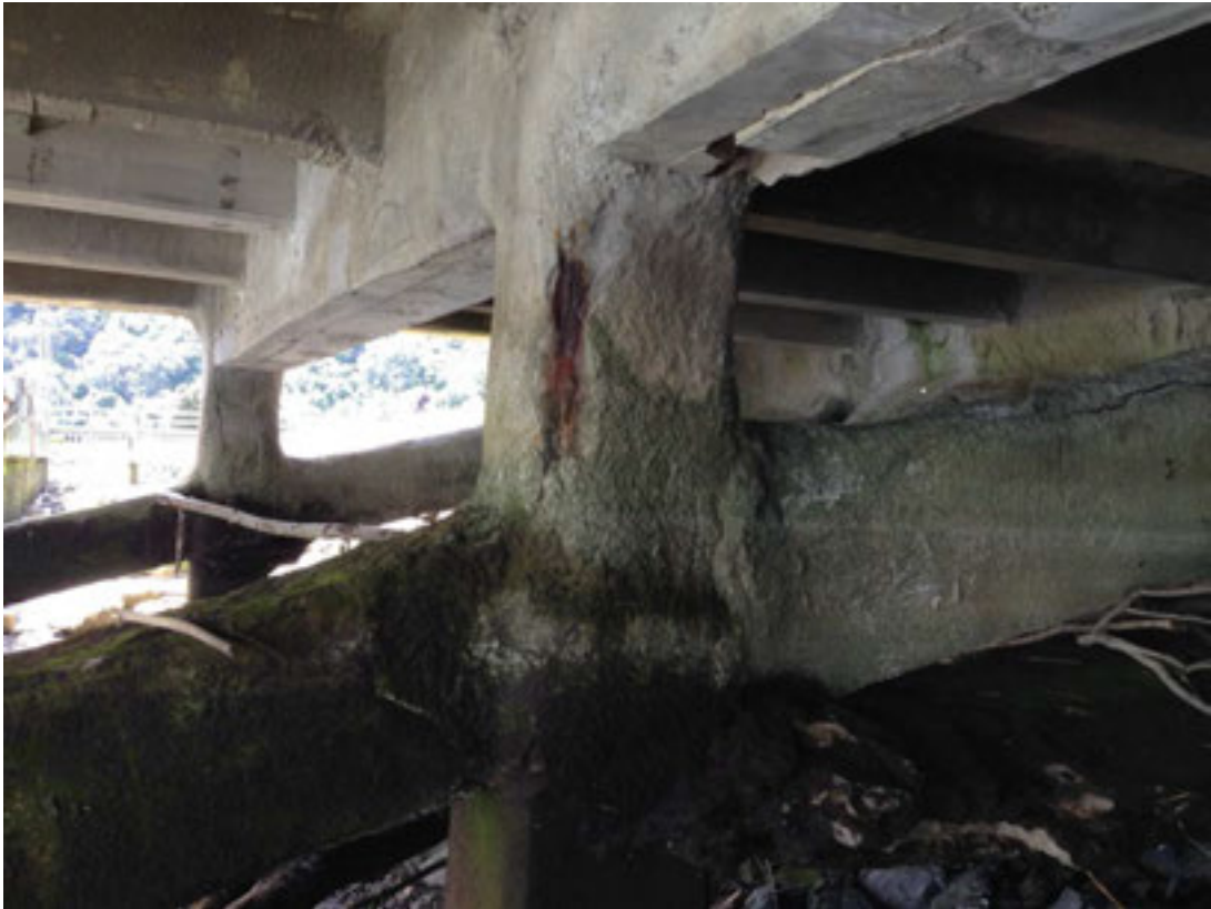
Photo A12 - spalling / corrosion at A2
