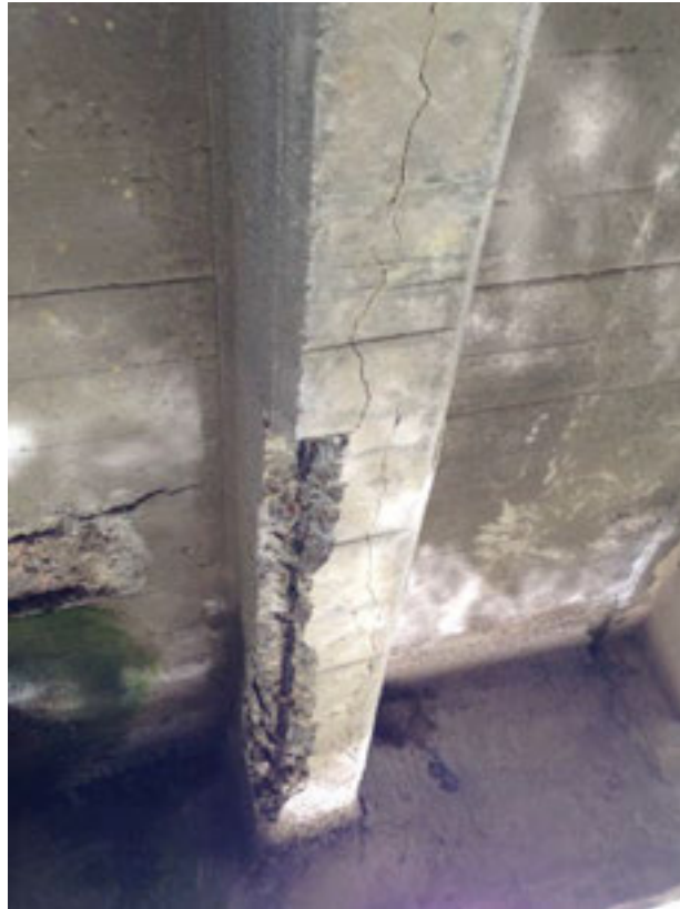
Photo A08 - beam cracking / spalling between A1 and A2
