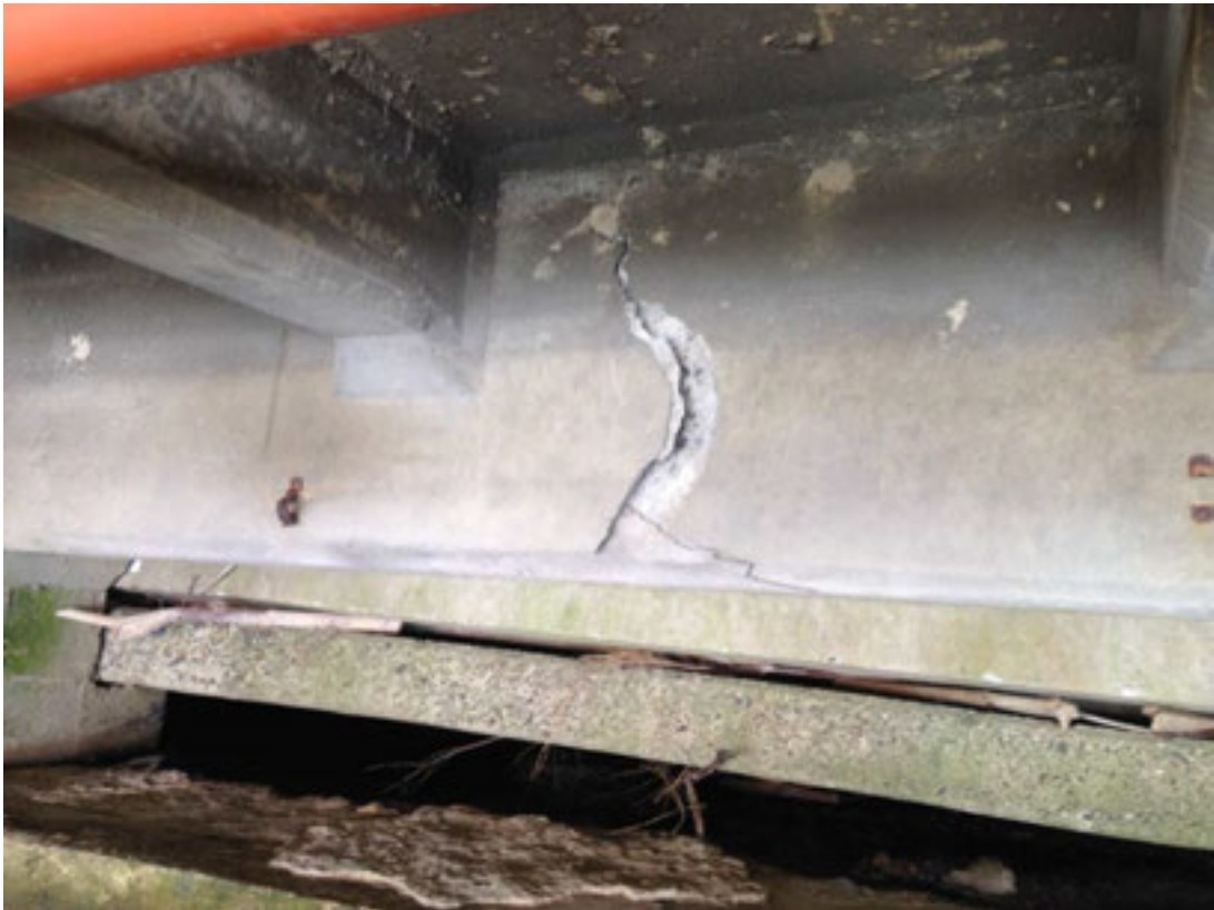
Photo B17 - cracking of rear beam between B15 and B16
