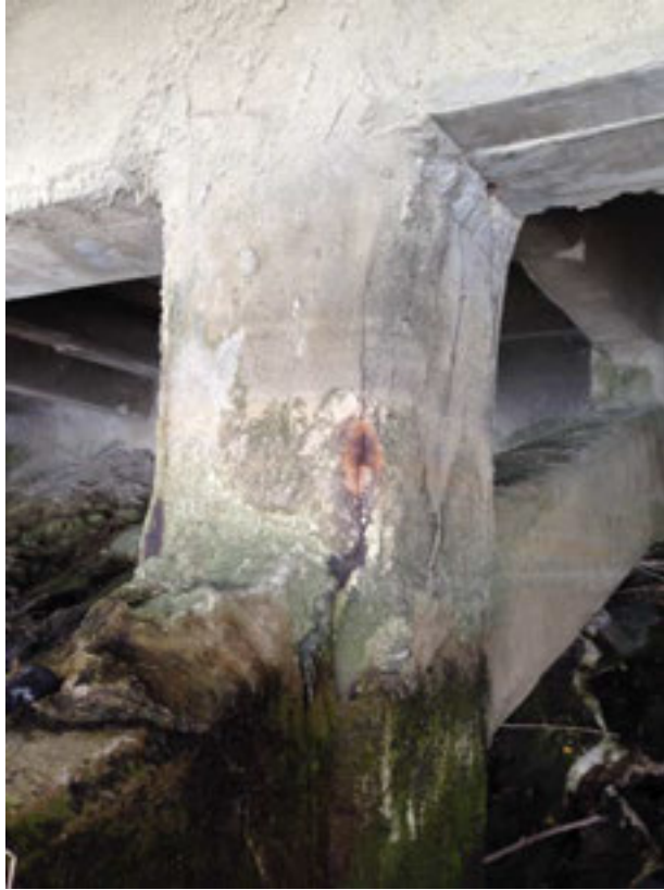
Photo A18 - Pile cracking at A3
