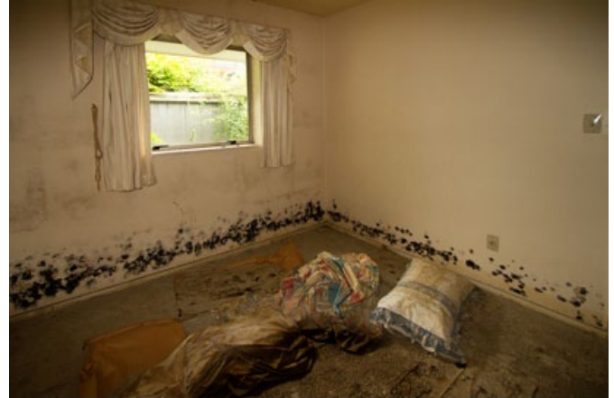
Figure 1: Interior of a Christchurch house affected by mould. This photograph was taken approximately eight months after the February 2011 earthquake.
