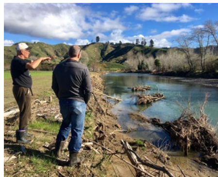
Kevin Clark explains the flood's effects to Simon Stokes from the Whakatāne District Recovery Project team. Note the extent of erosion behind the defence groynes.
