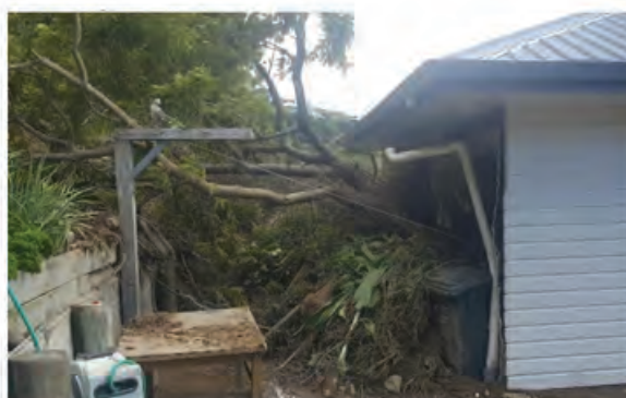
Figure 2 Landslide damage to garage wall
