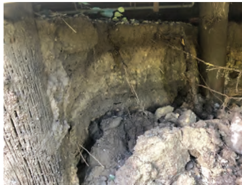
Figure 4 Erosion around driven piles
