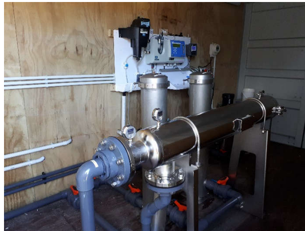
Figure 6: WTP Cartridge filtration and monitoring equipment within container housing
