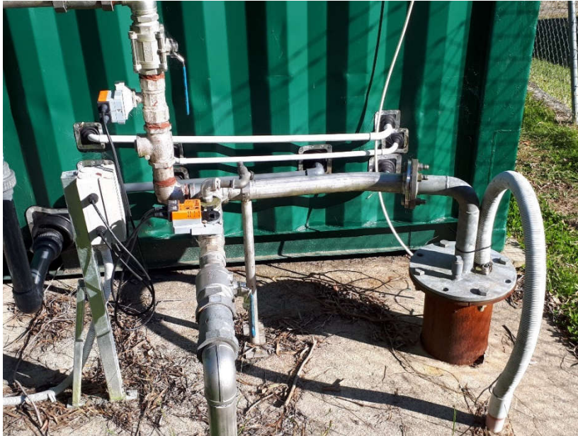
Figure 5: Bore Head Works at Pump Station/Treatment Plant Site
