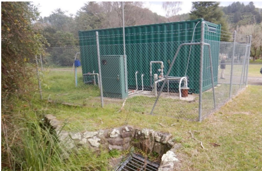
Figure 4: Bore Head and Container Housing for Treatment Equipment at Pump Station/Treatment Plant Site
